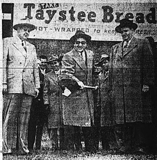
GROUND BREAKING CEREMONY —A shovel-full of earth is turned as the first step in a big, new building project being launched by the Taystee Bread and Grennan Cakes Company. With the shovel above (center) is Arthur H. Frost, the new Memphis manager for the company. Looking on are George J. Parson at left, regional manager for the Purity Bakeries Corporation and Trow W. Dadd, Chicago, assistant vice president of the company in charge of engineering.
