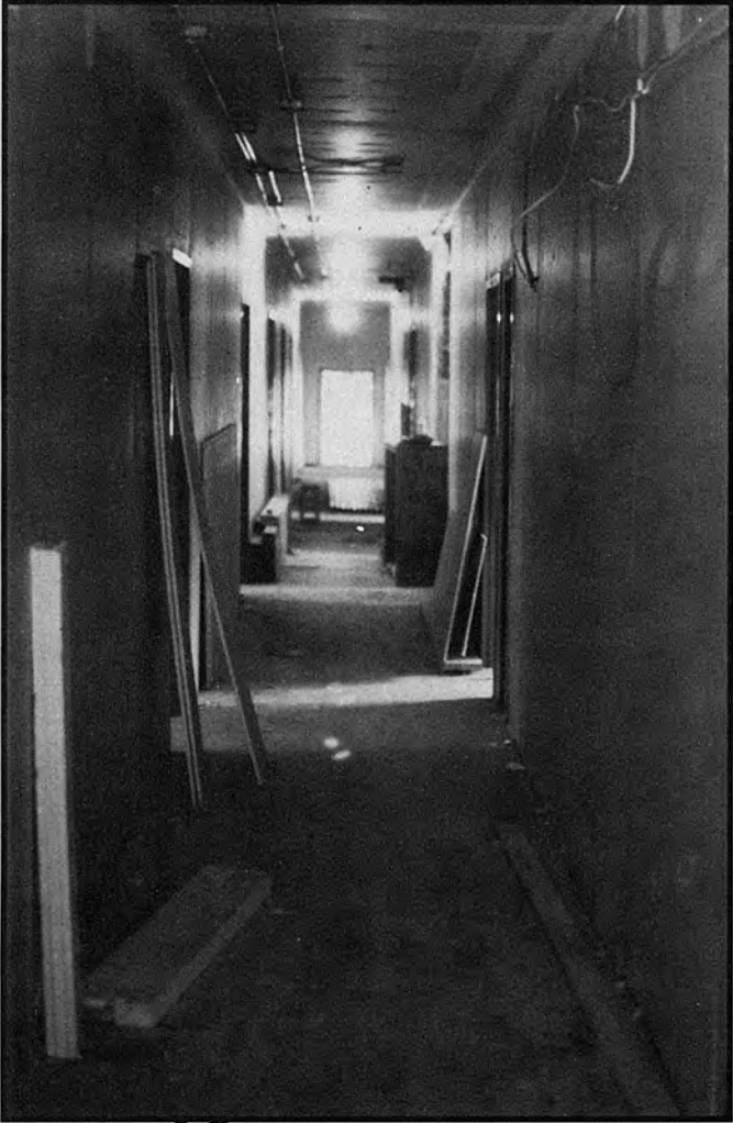
Stewart in the summertime. Changes on campus included renovations of Stewart Hall during the summer.
