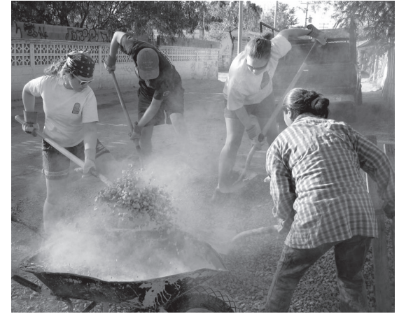
Student volunteers mix concrete to be used to help build 24 houses in Reynosa, Mexico.
