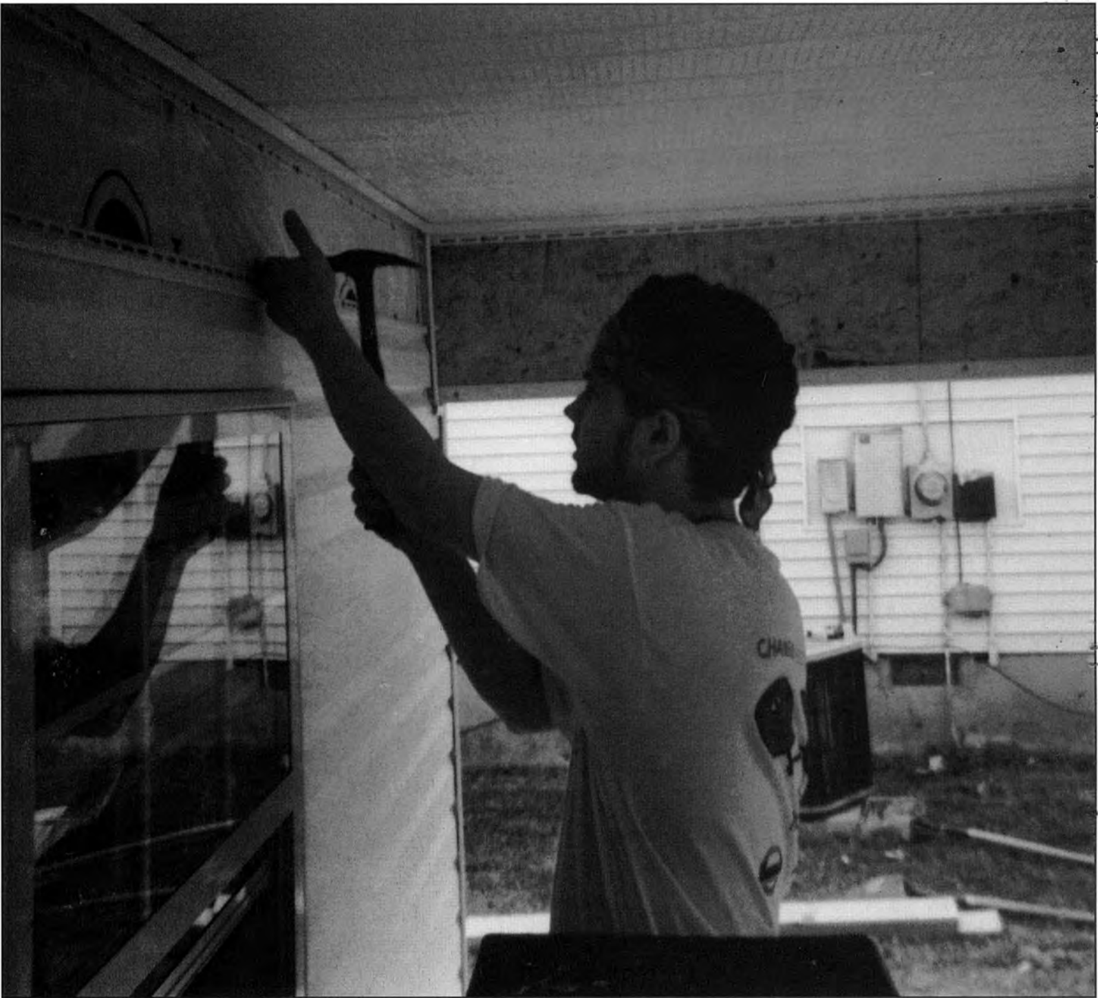
Above: Senior Josh Welter helps construct a house for Habitat for Humanity.
