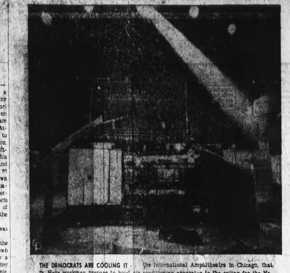
THE DEMOCRATS ARE COOLING IT -- the International Amphitheatre in Chicago, that in Here workmen prepares to hoist air conditioning apparatus to the ceiling for the National Convention opening Aug. 25. The units have a cooling capacity of 600,000 tons.
