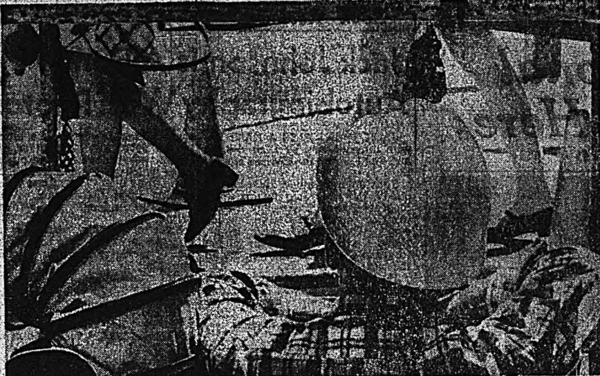
AHH... SPRING—On his way out of a manhole, this Southern Bell cable installer pauses to enjoy the benefits of summer along main street. There's been many a change in the scenery around the employee's office, and he appears quite satisfied with his ground level point of view.
