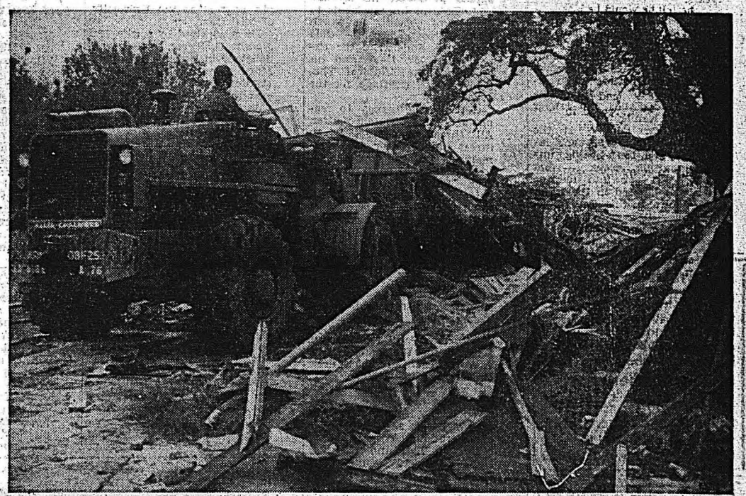
ARMY ENGINEERS of the 818th Engineer Battalion (Combat) clear rubble from a demolished building with a scoop loader shortly after hurricane Camille struck the Gulf coast in Mississippi. The 818th and the 48d Engineer Battalions were among
