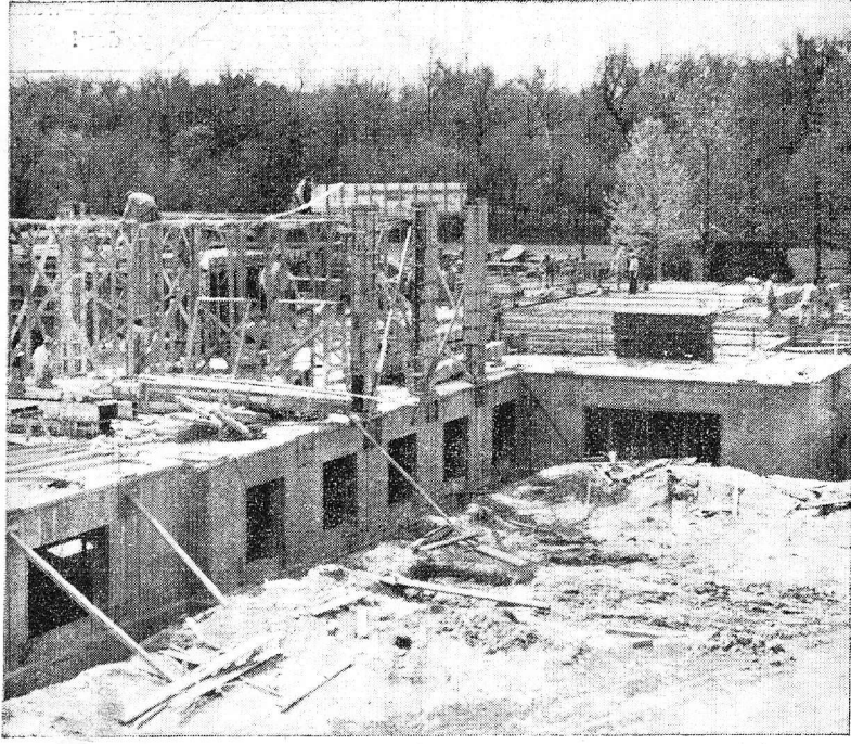
This is Burrow Library shortly after the foundations had been laid last year.
