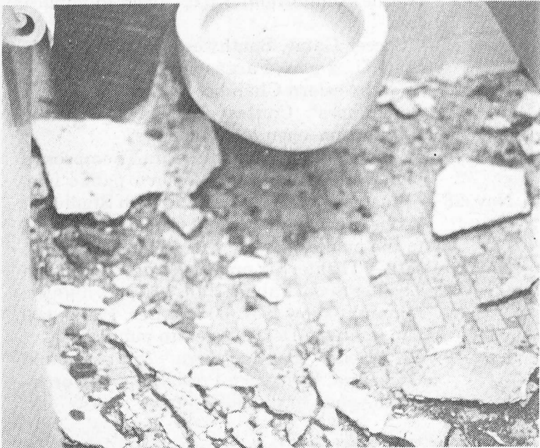
RENOVATION GOES DOWN THE TOILET. Plumbing problems caused the ceiling in the first floor Ellett bathroom to cave in earlier this week. photo by Joe Krakoviak
