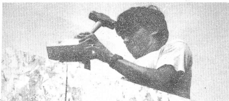
Ned Willard braces one of the walls of the Habitat for Humanity project house. Much progress has been made since the walls were raised. The house is now more than 50% complete.
