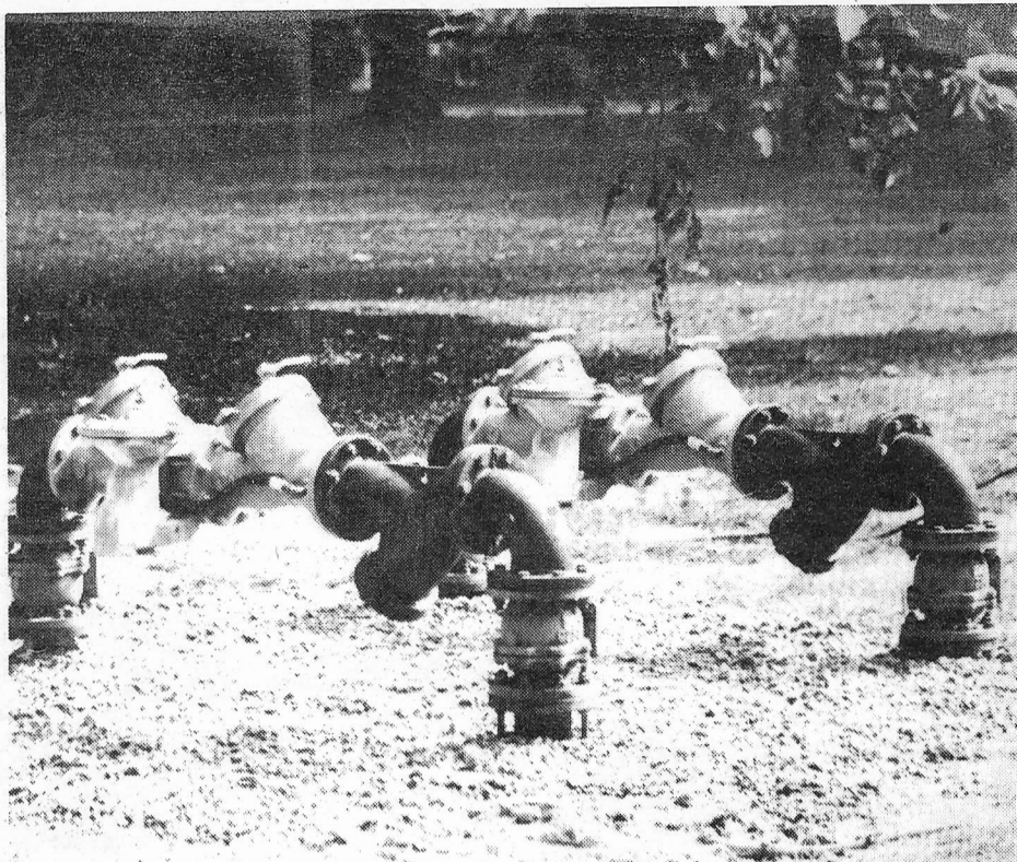
THE BIG BLUE THINGS. These aesthetic additions to Oak Alley are backflow preventers, fulfilling Shelby County code requirements by preventing College water from backing into city water mains. Plans to landscape are underway.
