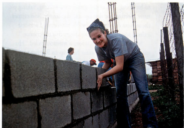
Meg Chambers smooths wet mezcla that she has applied between cinder blocks
