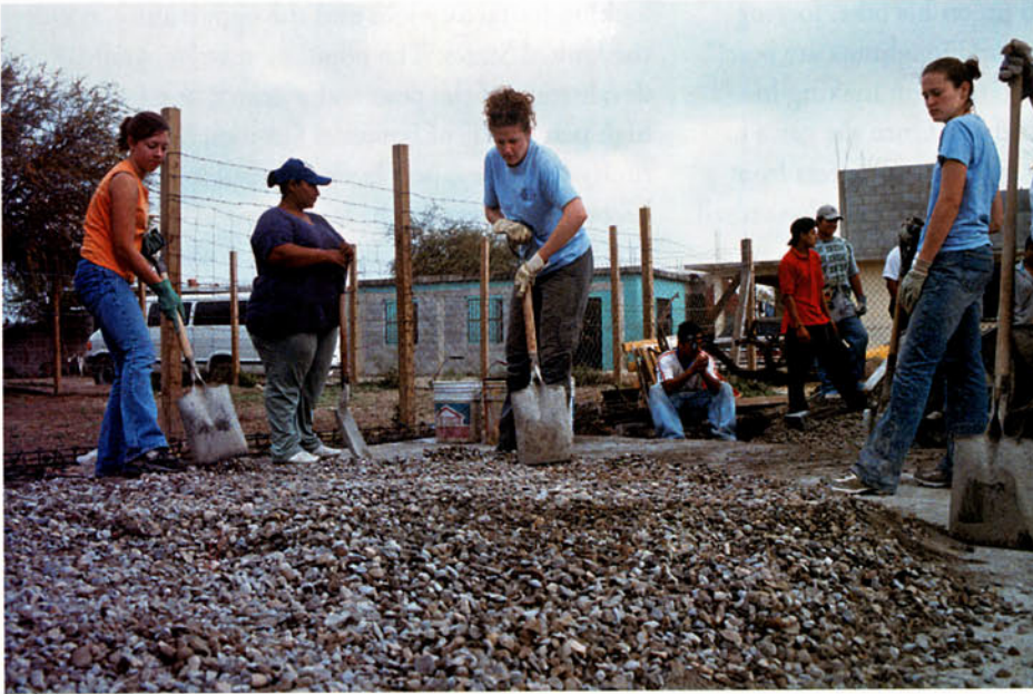
Ashley Carver '06 (left), Brooke Molpus '03 (center), Meg Chambers '06 and Ministerio de Fe volunteers toil at mixing mezcla , a combination of sand, concrete and water that cements the cinder blocks together to form a single-room structure. Even though the work is laborious and tough on the muscles, the volunteers joke, laugh and sing as they shovel the mix.
