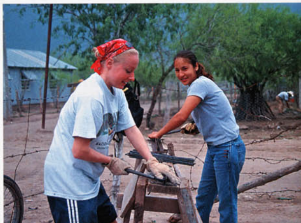
Elaine Odle '04 and Mexican volunteer fabricate metal rebar, used in columns that support walls and in grids that support roofs
